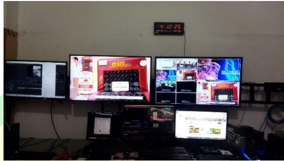
Gambar 3.16 Master Control Room (MCR) Sumber : Dokumentasi Peneliti
